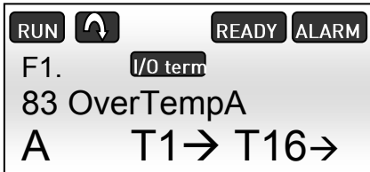
Figure 7.1-2, High temperature alarm on the NXP panel
