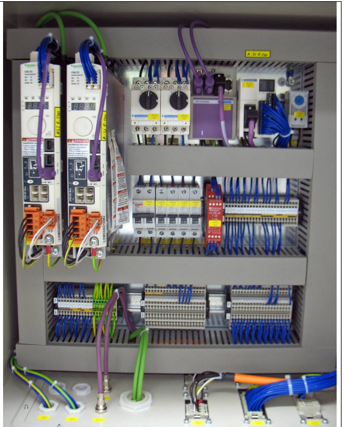
Distributed cabinet H3 & H4 Interior
