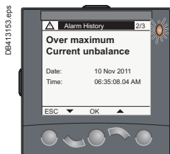
Phase unbalance alarm.
