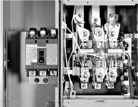
Q-Frame Circuit Breaker Installed
