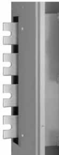
Left End of 3Ø Horizontal Cross Bus, Shown with Slotted End Bus Bars
