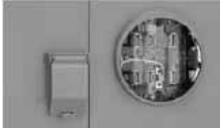
BCV Circuit Breaker Door Shown with Door Closed
