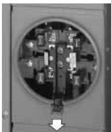
Manual Slider-Type Bypass Shown in Closed Position with Handle Extending through Notch in Rim of Meter Socket Cover
