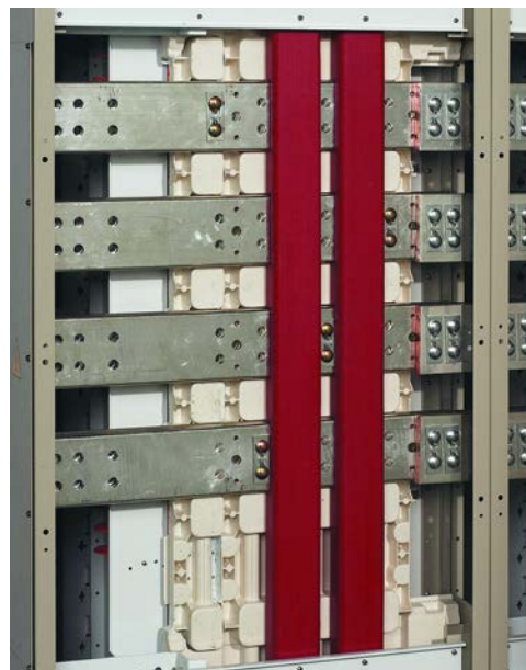
Horizontal and neutral bus at back of MCC unit (back plate of MCC unit removed)
