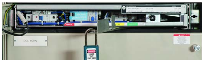
Withdraw lever in the Test position (and locked out).
