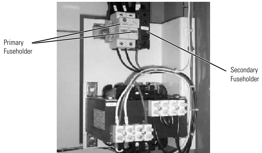
Figure 5.14 Checking the Wiring and Fusing of the Control Transformer
