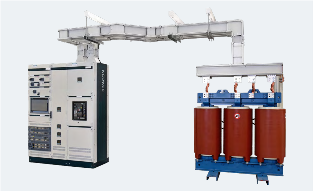
Fig. 2/2: Connection of a transformer to a Siemens power distribution board
