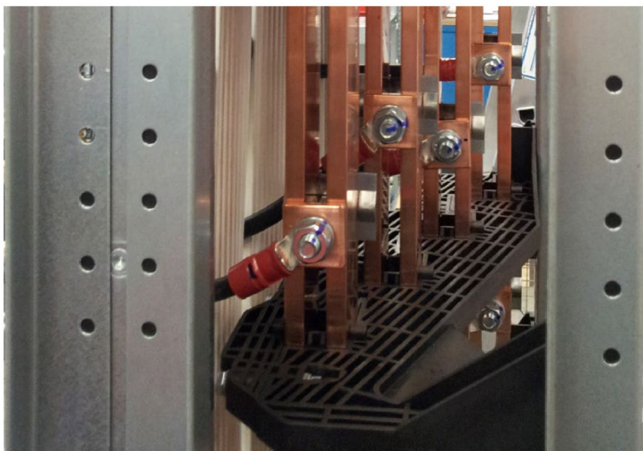
Connection to vertical busbar system
