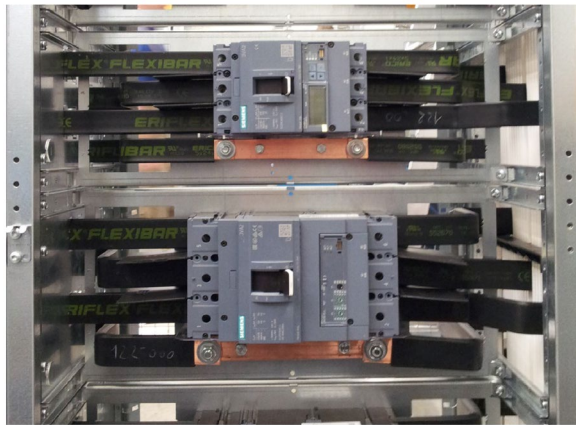
Connections in the compartment in form 3B with terminals
