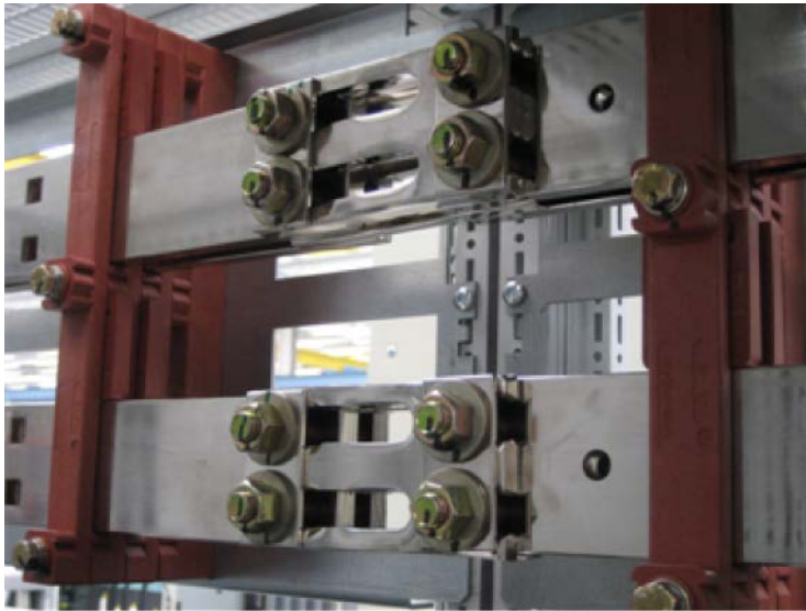
Figure 9-39 M80 - M87, DC busbar
