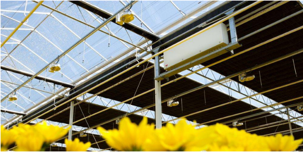
02 Example for the position of a lamp starter cabinet in a horticultural greenhouse
