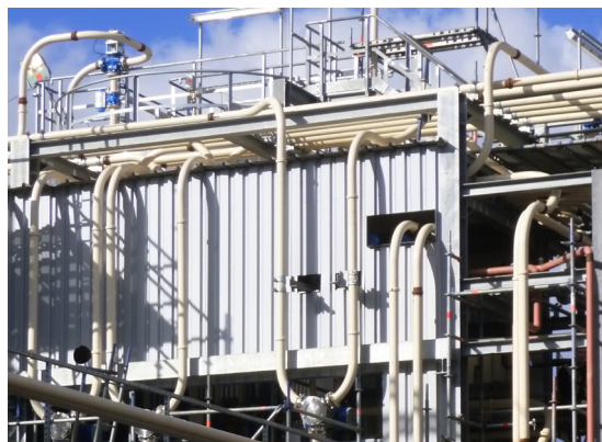
Pigged lines with diverter and distribution valves
