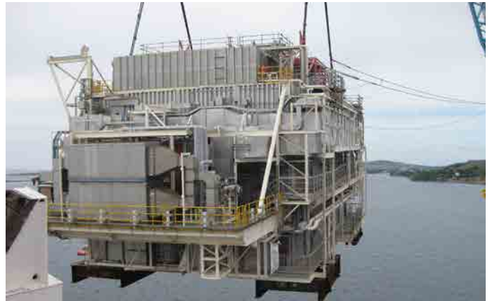
Figure 2: HVDC - Light Station VailHall
