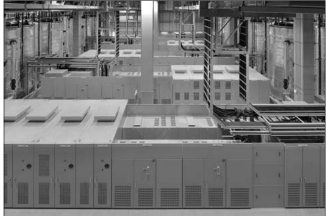
Fig.2 Installation status of power conditioning equipment
